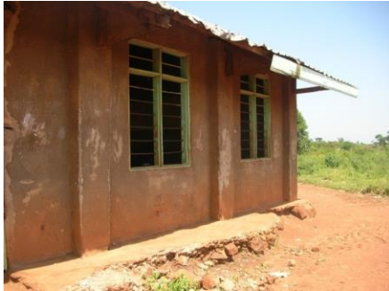
Plate 5.7. Iron sheets destroyed by lightning at Runyanya Primary school.
