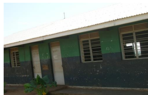
Plate 5.8. Installed lightning conductor at one of the roofs at the school.
