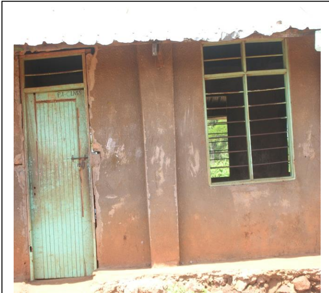
One of the building in Runyaya school that was struck by lightning
