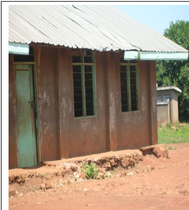
A school roof at Runyaya P.S that was struck by lightning.
