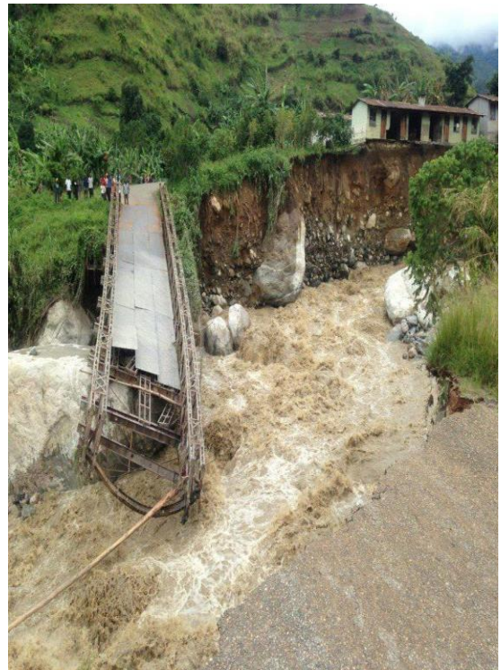
Houses hanging dangerously at the river bank in Kilembe after the floods.
