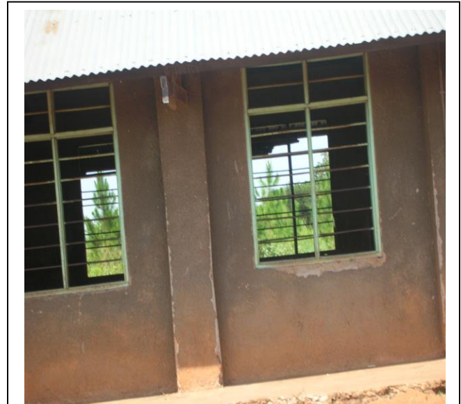
Open windows in the class room at Runyaya P.S. This could have contributed to the pupils being struck.
