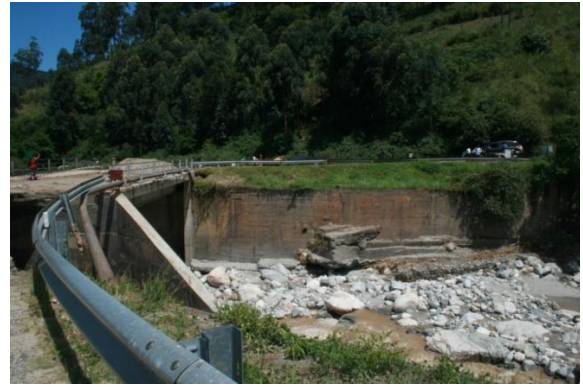
Plate 2.5: A bridge damaged at Kilembe town. Photo credit; Kitutu Goretti
