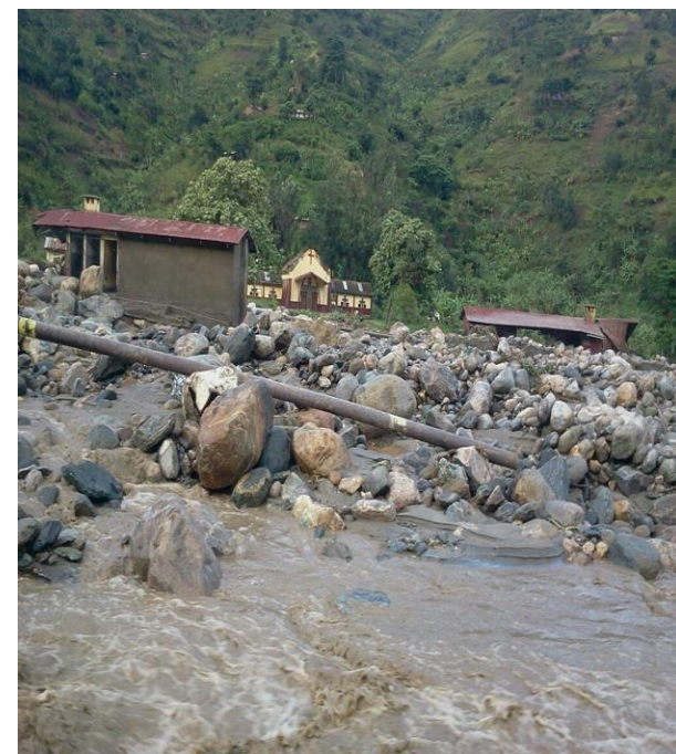
Broken pipes among debris brought by floods
