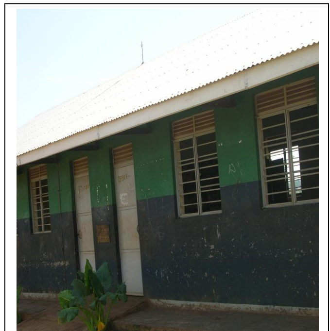
Lightning conductor on top of the roof at Runyaya P.S
