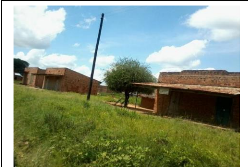
Plate 5.3 Houses that were struck by lightning killing three persons in Bukedea District.
