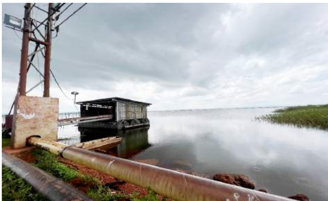
Photo showing the pumping station at the shore of Emin Pasha gulf at Nungwe port
